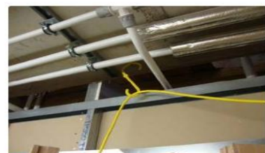
Cables suspended using proprietary hooks to prevent trailing cables on floor area.
