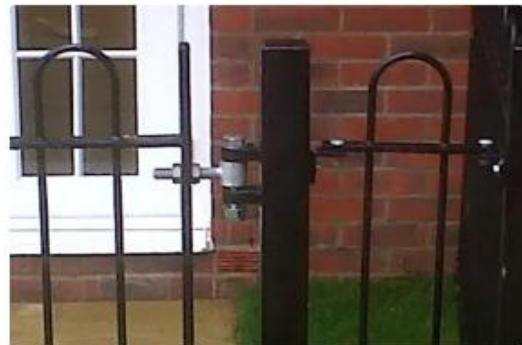
Note the modified hinge with adequate space between gatepost and pillar
