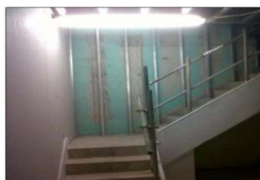
No trailing cables in the stair core.
