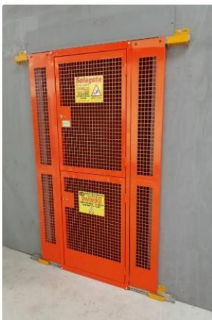
Lift shaft protected with proprietary full height safety gates
