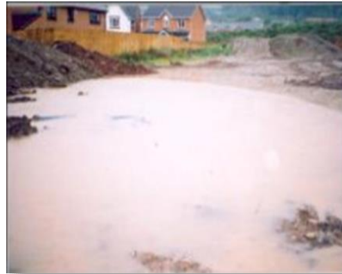
Excessive/unnecessary soil strip
