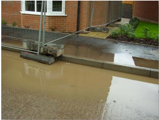
Result of Terram (Drains) not maintained
